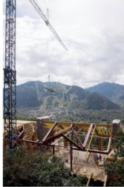
Construction continues on a 15,000-square-foot home on Red Mountain, overlooking Aspen and the town's ski hill. The average single-family home in Aspen measures 3,272 square feet. (Special to The Post / Zach Ornitz)
